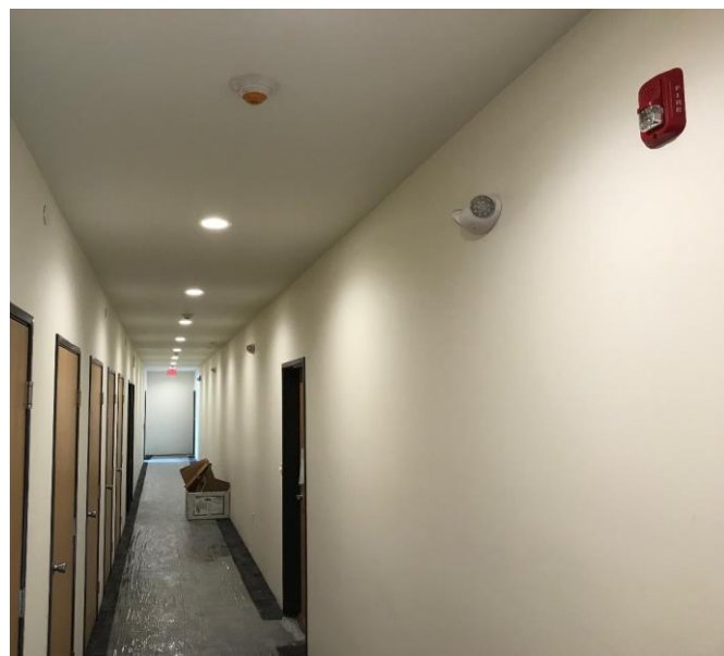
Notification Devices - Horn/Strobe, Smoke Detectors, e-Lights
