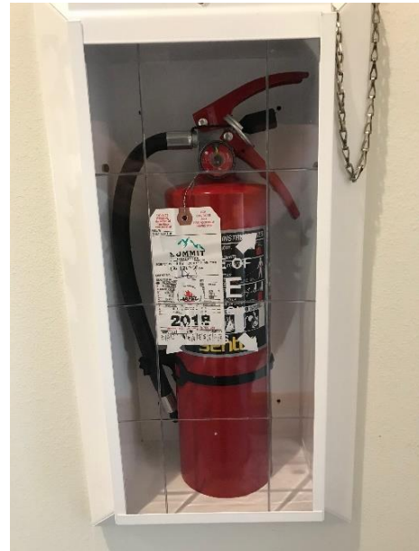
Hand Portable Dry Chemical Fire Extinguisher
